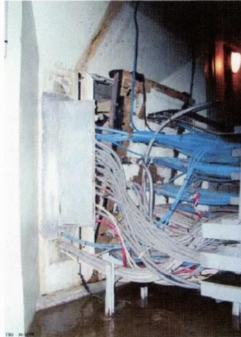
Failure of Cable opening
